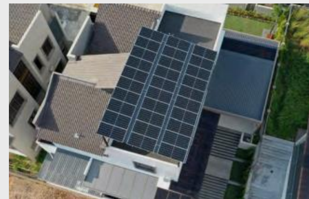
Sungai Petani, Kedah 17.35kWp
