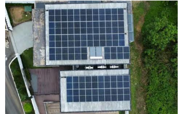
Kuala Krai, Kelantan 17.54 kWp
