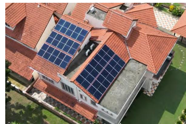
Shah Alam, Selangor 16.68kWp
