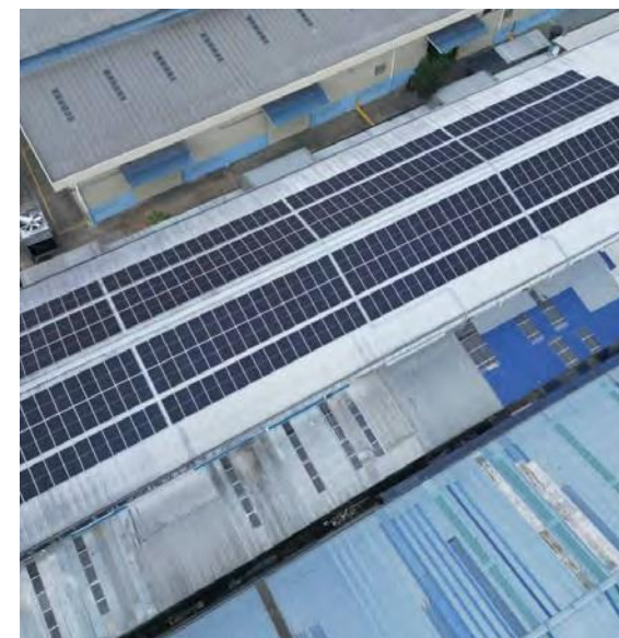
PLATINUM VEST SDN BHD [ Property Investment & Leasing ] 220.98kWp, Sg Buloh, Selangor
