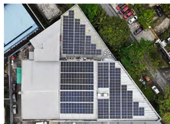
UNITED YL PRINTERS SDN BHD [ Printing Services ] 133.315kWp, Kepong, KL
